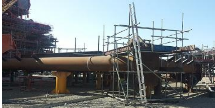
Figure 7. Rust grade B.
